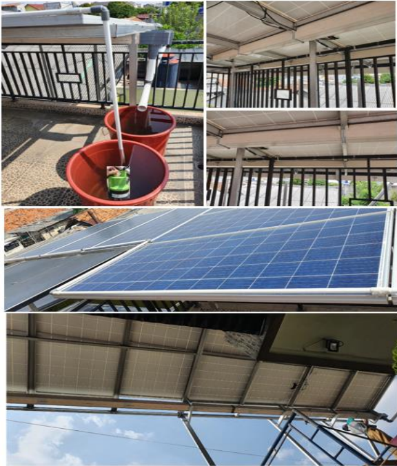
Figure 3. Installed cooling system
