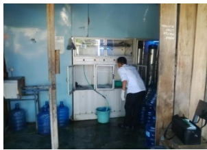
Figure 3. Floors that do not meet the requirements because there is stagnant water. Depot floors must be waterproof, flat, smooth, not slippery, not cracked, does not absorb dust, and is easy to clean, and the slope is sufficiently gentle to ease cleaning and no standing water.
