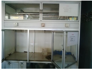
Figure 2. Leakage in the Depot Faucet: the leakage in the depot faucet increases bacteriological contamination of drinking water, this is due to the water coming out of the mouth of the depot pipe becoming moist and allowing the growth of bacteria.
