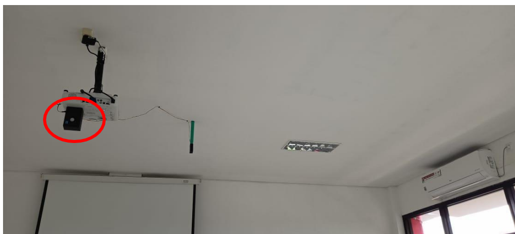
Figure 4 Device Position in Classroom
