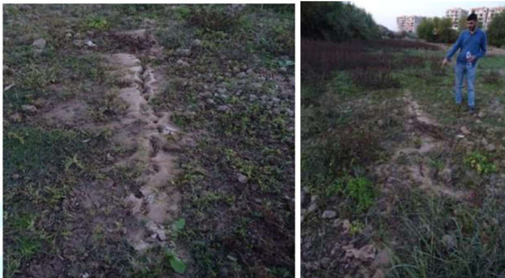
Figure 9. Images of the liquefaction phenomenon and sand boiling in different parts of the riverbed near Shahid Shiroodi Mehr housing complex (IIEES, 2017).
