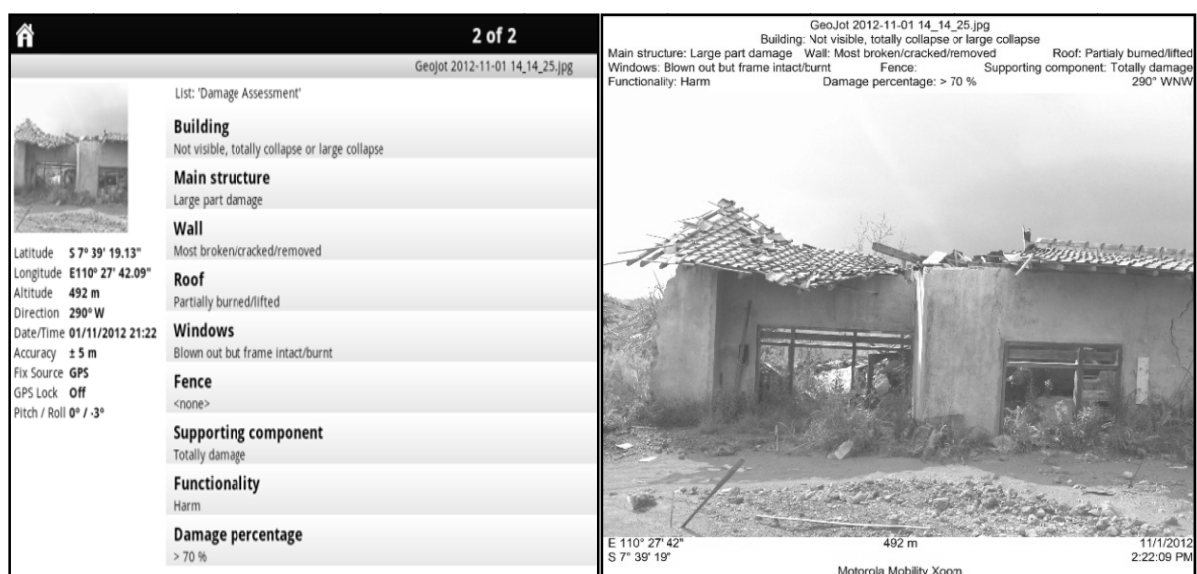
Figure 5. Building damage interpretation in Geojot (left) and its interpretation report from Geojot to GPS Photo Link (right).
