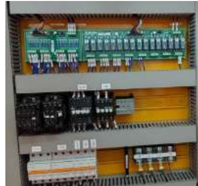
Gambar 5. Panel Listrik 3 phase 220v
