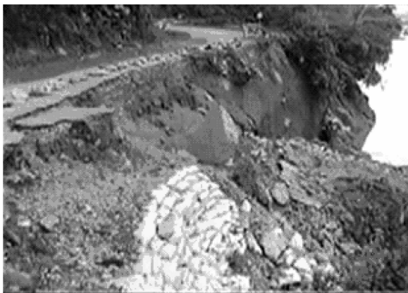
Figure 9: Landslide found in Chaungkyin area
