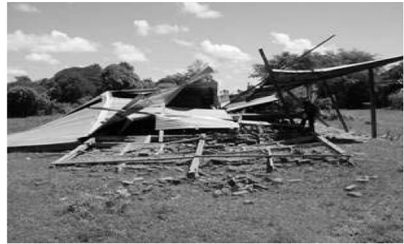
Figure 2: Collapse of primary school at Chezeing village during Taungdwingyi earthquake
