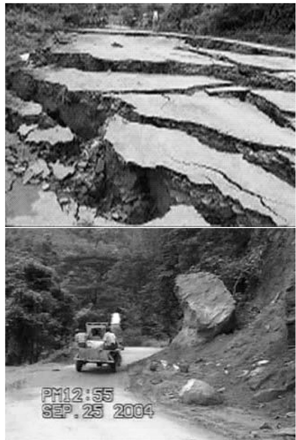
Figure 10: Serious landslides and rock- falls along Kale-Kalewa main road
