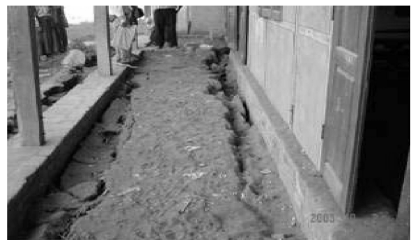
Figure 3: Settlement of school foundation due to liquefaction
