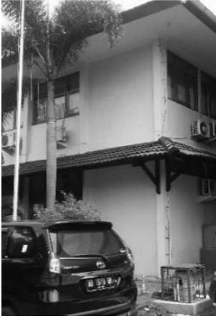
Figure 2. Rainwater gutters without vertical pipes at Serayu Opak River Basin Organization building.
