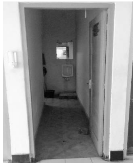
Figure 5. Location of the urinal in PJSA and Water Resources Field (WRF) building facing corridor.
