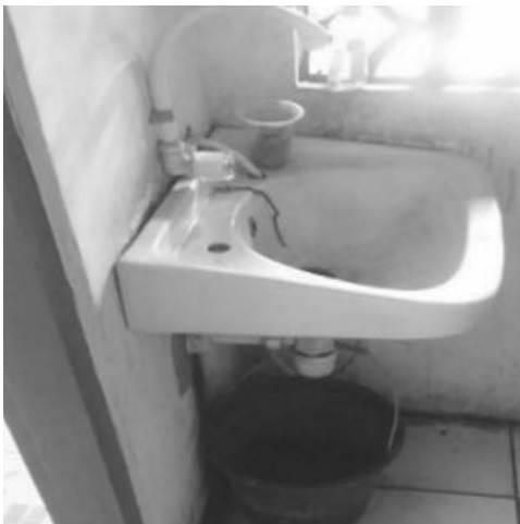
Figure 3. The location of the sink in the Water Resources Management Centre (WRMC) building.
