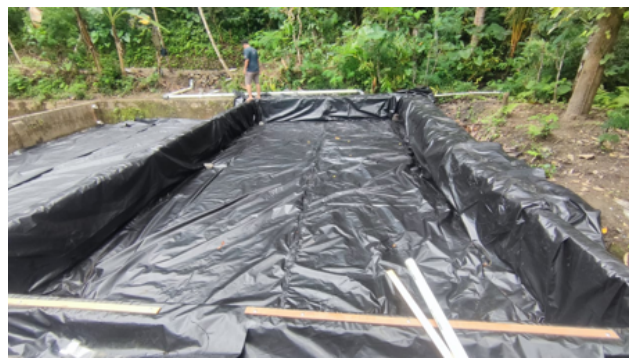
Figure 5. Use of geomembrane for fishpond revitalization. The fishpond will have another function as a water retention pond during the extreme rain and flood on the Winong River.
