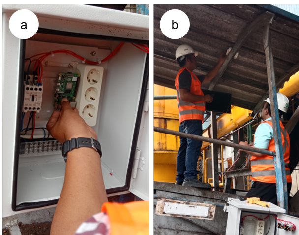
Figure 1. The installation of EFB count station creation: (a) Preparing a panel box for Raspberry Pi web server; (b) Installation of infrared sensors at the ends of the connecting plates between conveyors
