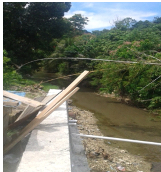
Gambar 3. Tanggul belum selesai Figure 3. The embankment has been not finished
